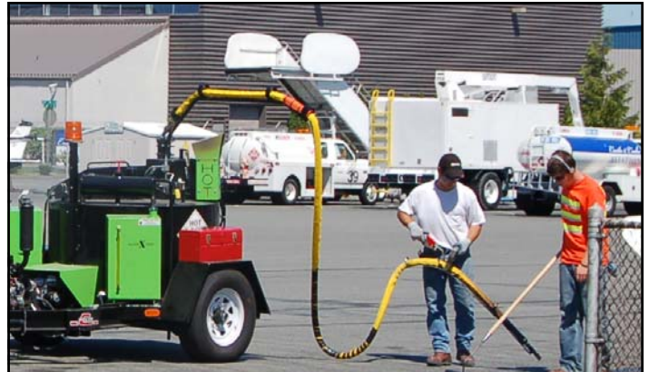
Airport Maintenance employees James Jamieson and Justin King are sealing cracks on the Central ramp.
